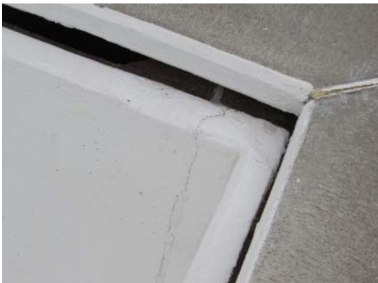
Vertical cracking along gutter and pool wall
