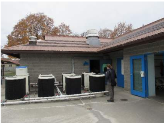
Heat pumps on pool deck
