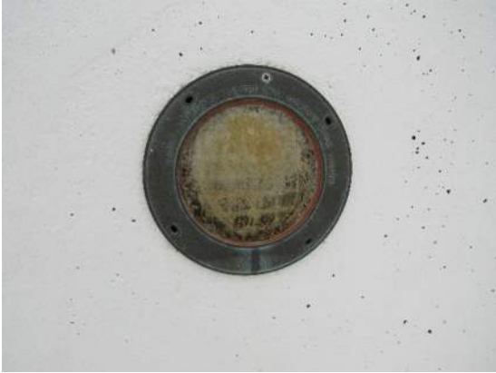
Underwater light with corrosion and mineral buildup
