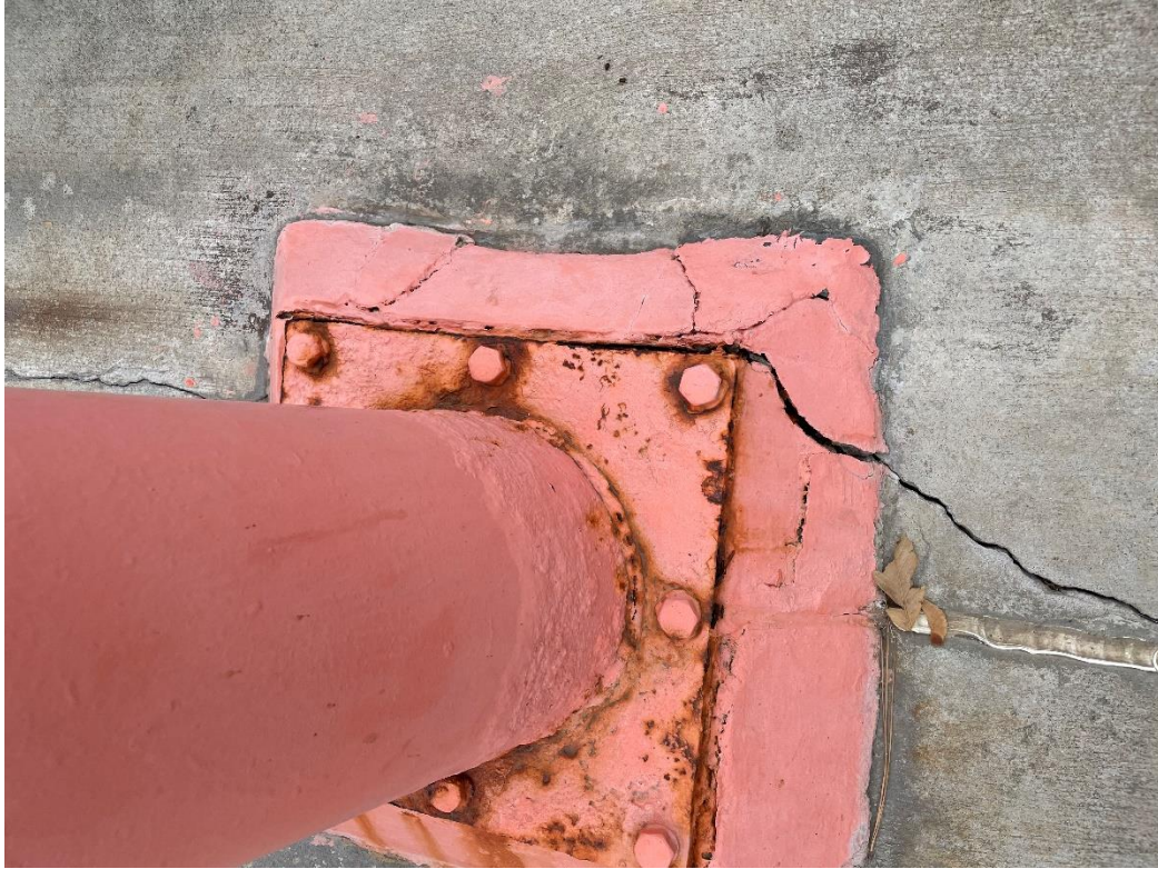
Plate 11 – Concrete Crack at Diving Board Mounting Plate
