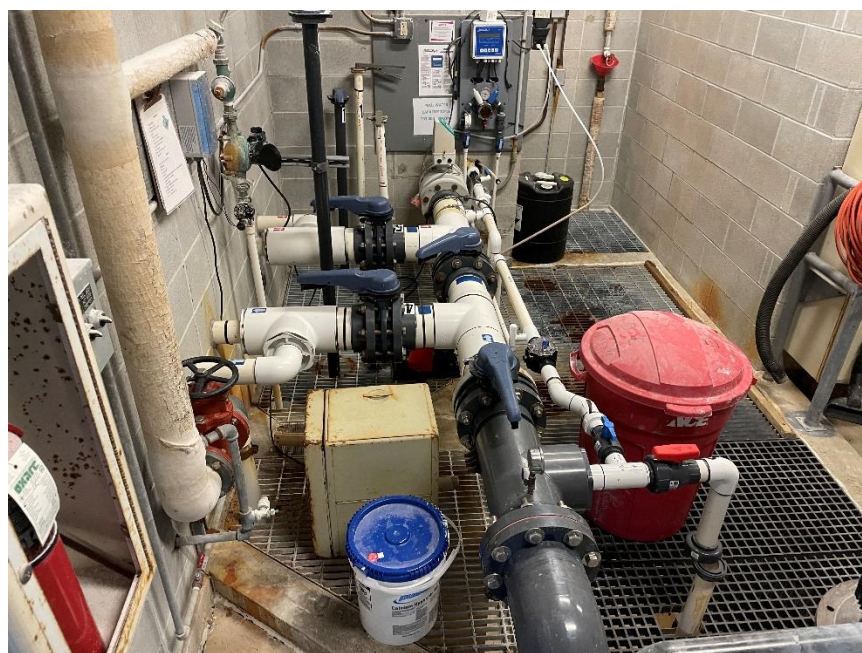
Plate 10 – Corroded Grating Panels
