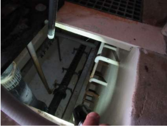
Vacuum DE filter tank with DE grids removed
