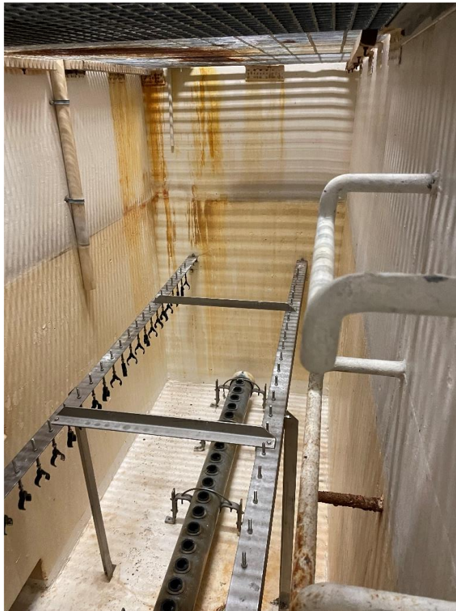
Plate 20 – Vacuum DE Filter Tank
