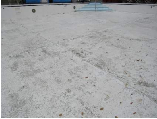
Floor of pool in shallow area, deteriorating paint finish
