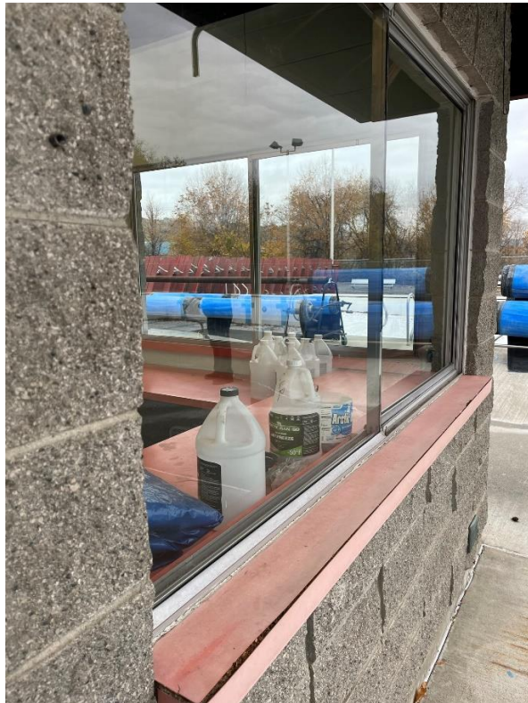
Plate 4 – Exterior Window Sill Delamination
