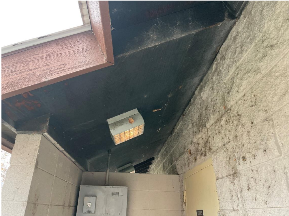
Plate 1 – Exterior Wood Fascia and Soffit Peeling Paint
