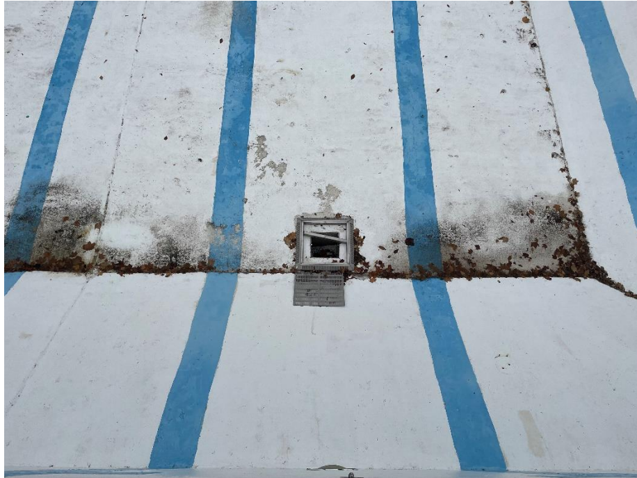
Plate 19 – Main Drain with Retrofit Cover
