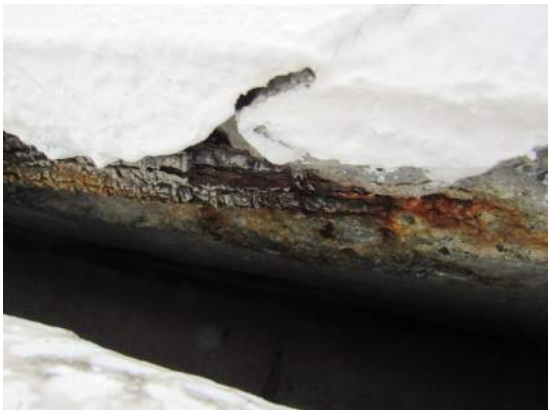
Spalling in gutter with exposed and corroded reinforcement
