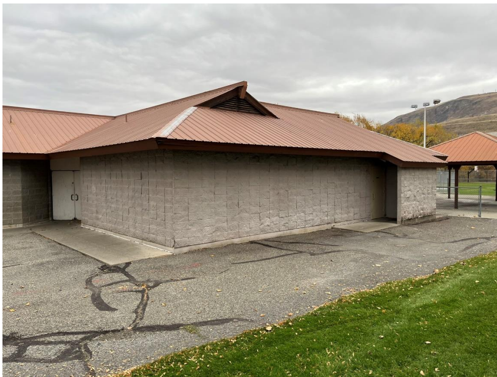
Plate 2 – Metal Roofing Oxidation
