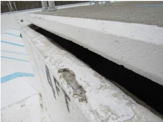
Gutter edge with spalling concrete
